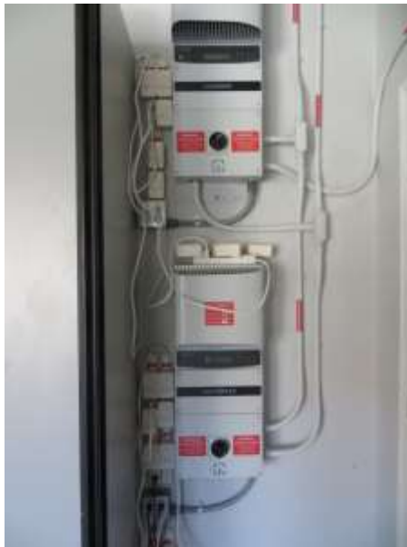
Figure 3 Solar Inverters with filters.
